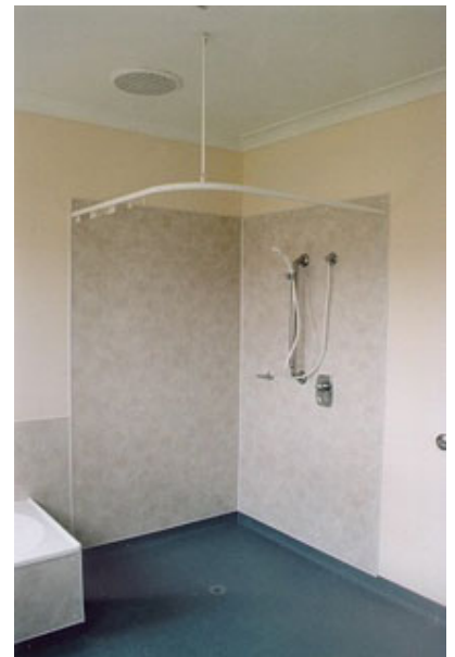
Disability Modifications Stepless Shower base. (Disability Modifications, 2007)
